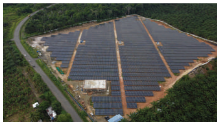
Large-Scale Solar Project, Tawau
