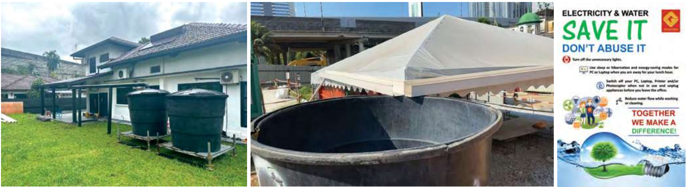
Rainwater harvesting system installed at RTS Link
